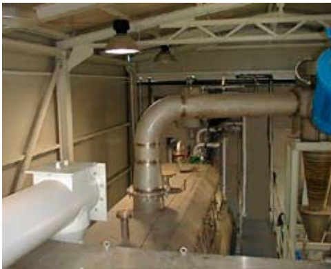
Rotadisc dryer with wet sludge intake to the left and cyclone to the right
