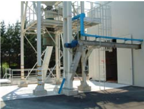
Dried sludge system with bucket elevator. Wet sludge intake hopper in the background
