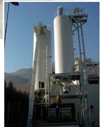
Plant with silo for wet sludge to the left and dried sludge to the right
